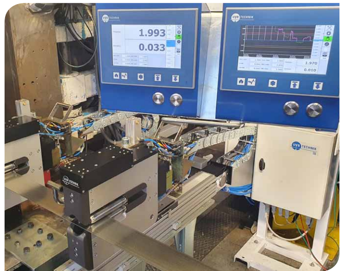
Tenneco, Italy, bimetal, rolling mill - Single line gauge + scanning head
